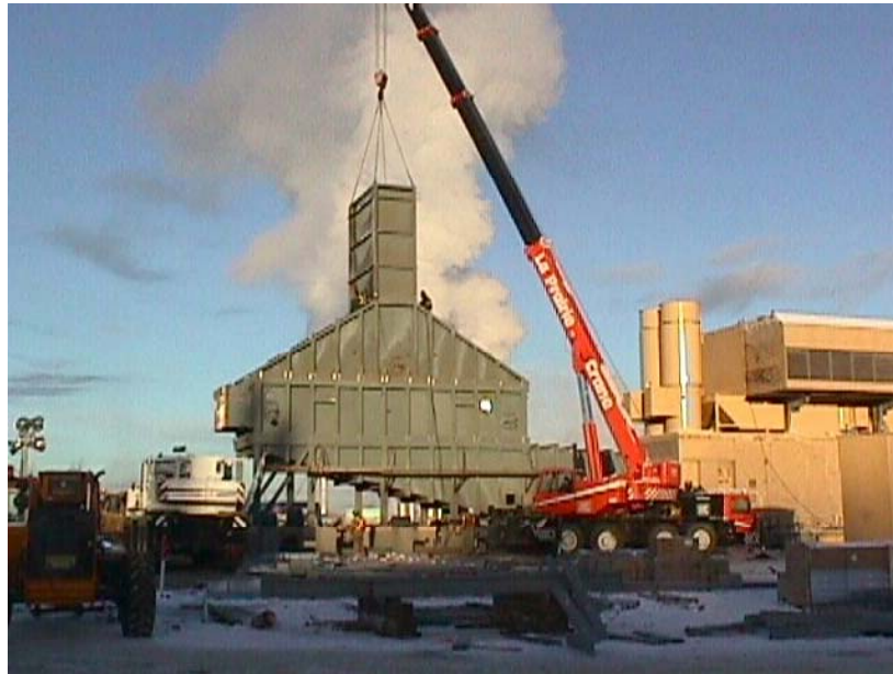
Figure #4 ñ Horizontal Tube/Vertical Gas Flow Arrangement LM6000PC Gas Turbine
