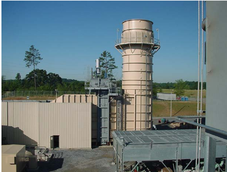
Figure #6 ñ Vertical Tube/Horizontal Gas Flow Arrangement Frame 7FA Gas Turbine
